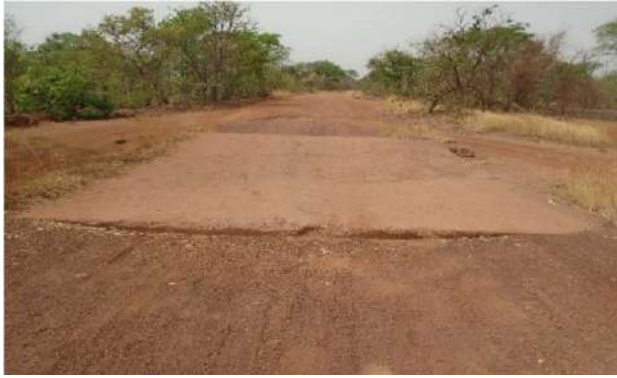
Photograph 5: Degraded surfacing (Source: APS report, 2021)
