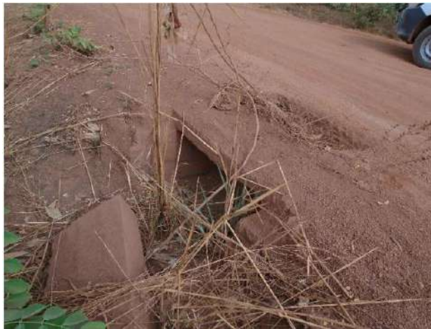
Photograph 7 Old gutter in poor condition (Source: APS Report, 2021)
