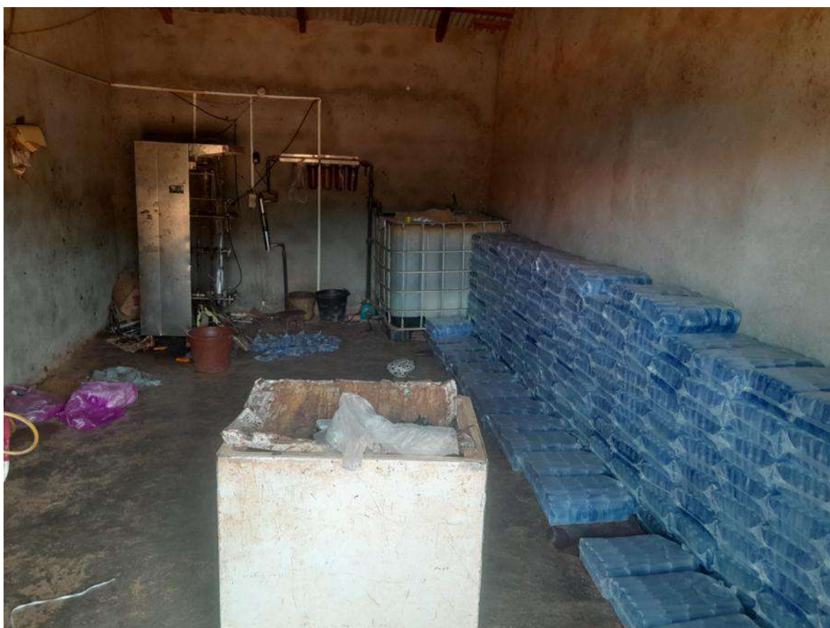
Photograph 50 : Water production plant, Source: Insuco, 2025
