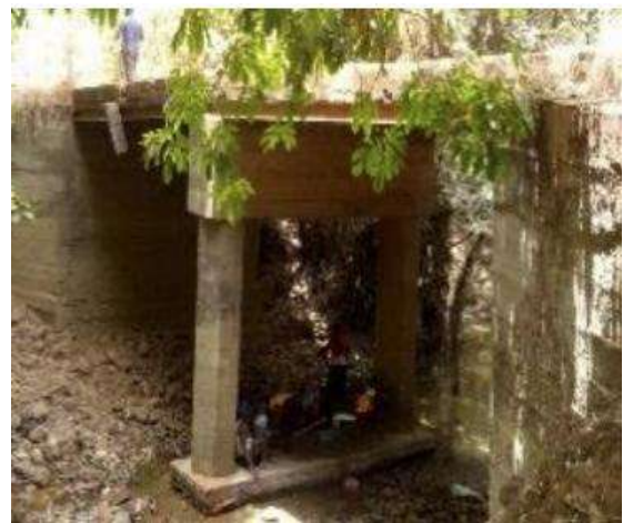
Photograph 8: Bridge undersized (Source: APS report, 2021)
